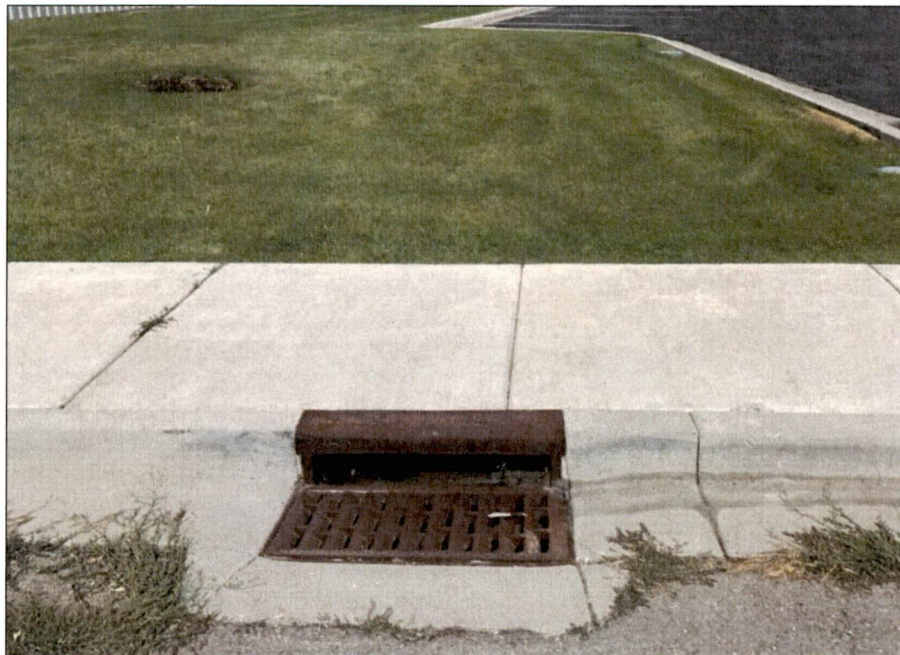
Figure 4. Incorrectly Oriented Directional Grate
