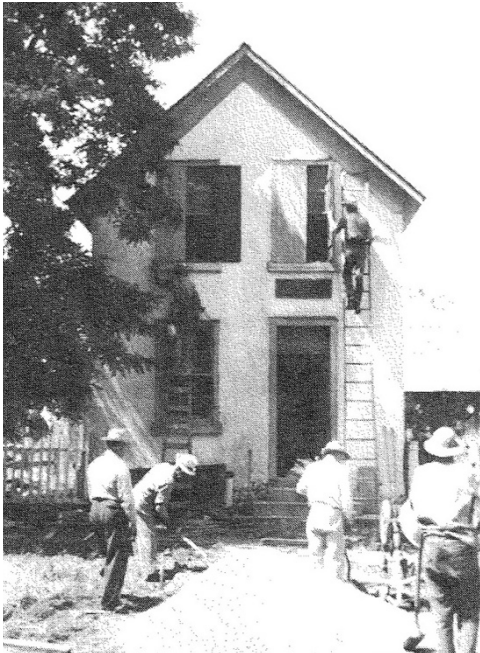
Figure 13. Work day at the Tithing Office to convert it to the Bishop's Storehouse in the 1950s. Credit: The Church of Jesus Christ of Latter-day Saints and Santaquin Utah Stake 1984, 12.
