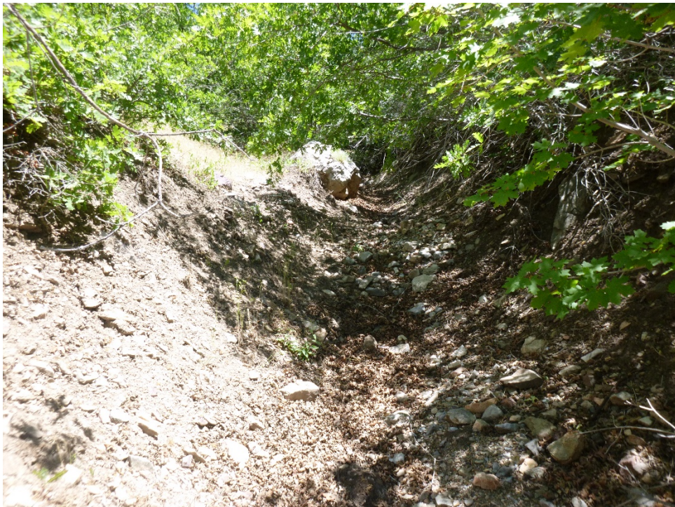
Figure 10- Depression near outflow location 1
