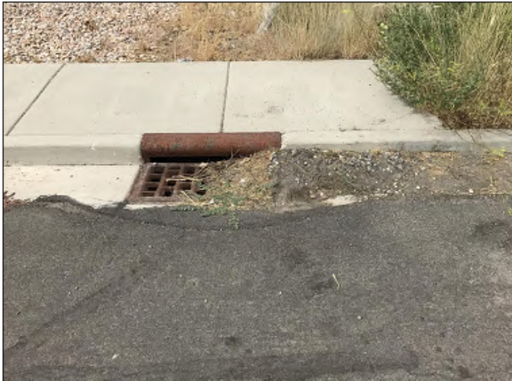
Figure 2. Inlet with Debris
