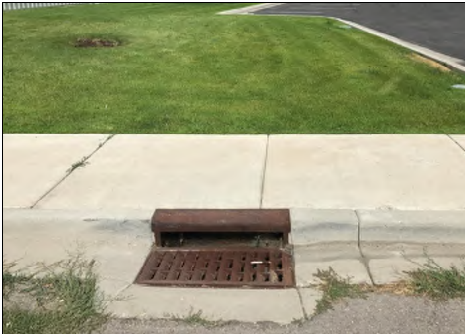
Figure 4. Incorrectly Oriented Directional Grate
