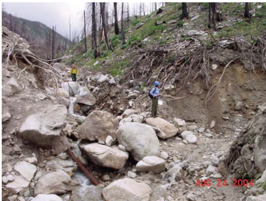
Figure 7. Channel incision from passage of debris flow in Lake Creek tributary to the Middle Fork Boise River. Photograph by Dave Hilgendorf, U.S. Department of Transportation Federal Highway Administration.
