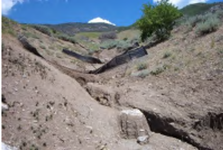
Figure 4. Failed silt fences near Farmington, UT.
