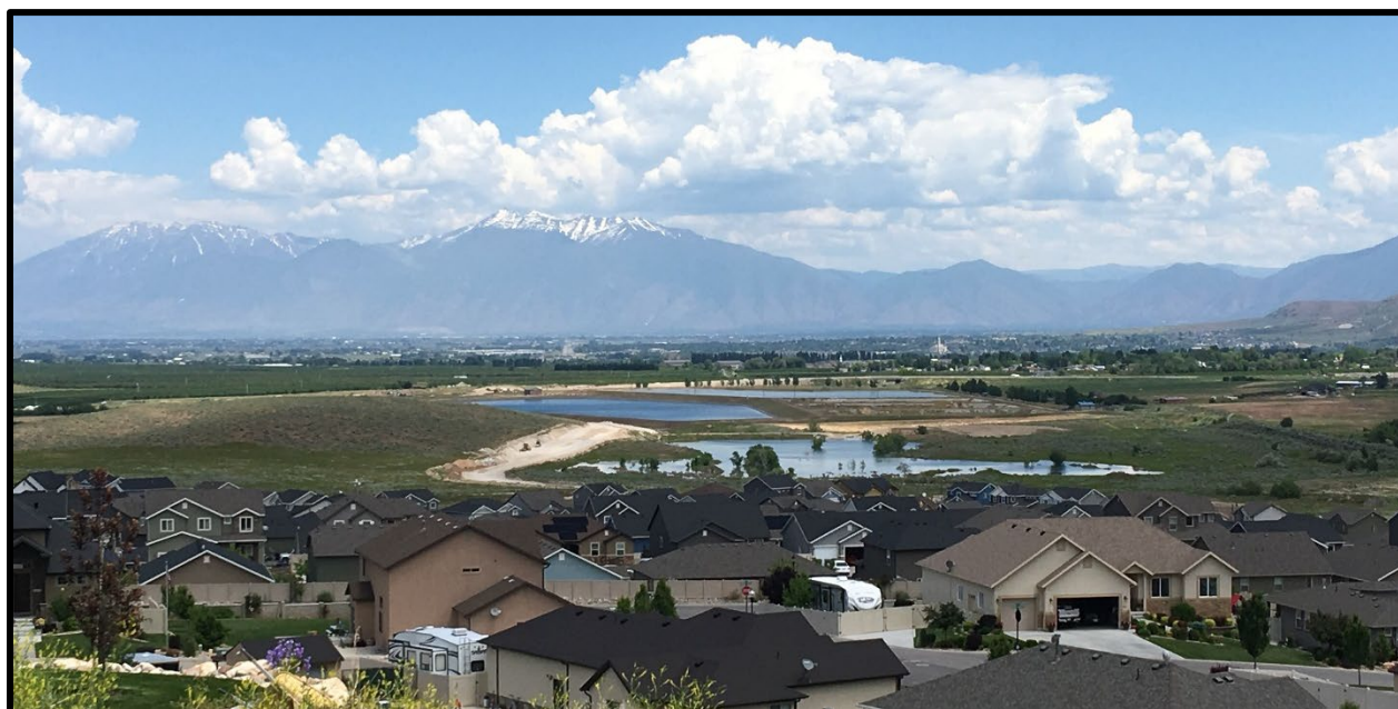
Extension of Summit Ridge Parkway to US-6 Main Street Under Construction – June 2019
